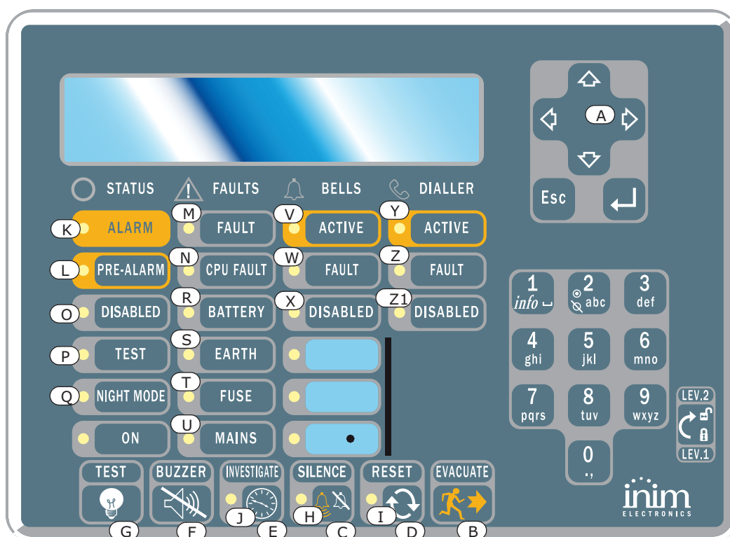
Figure 7 - Front view of the Repeater panel
